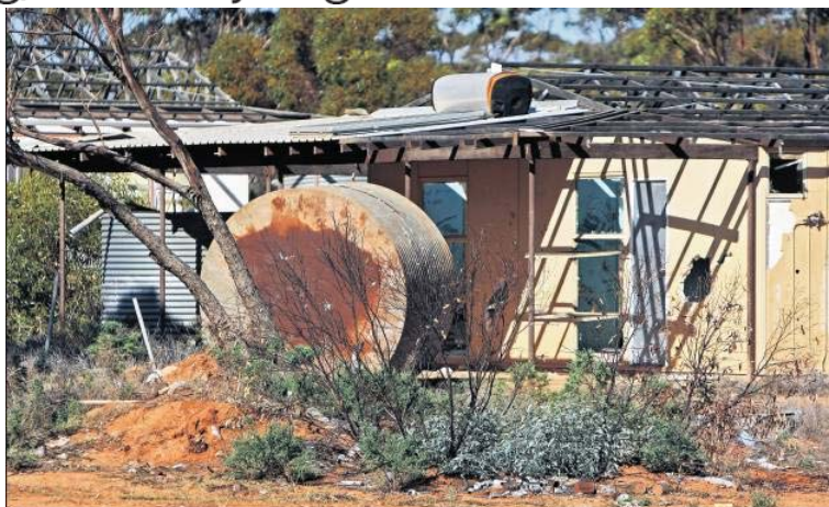
Substandard: Housing in many of WA's remote Aboriginal communities is substandard, according to a new report.
